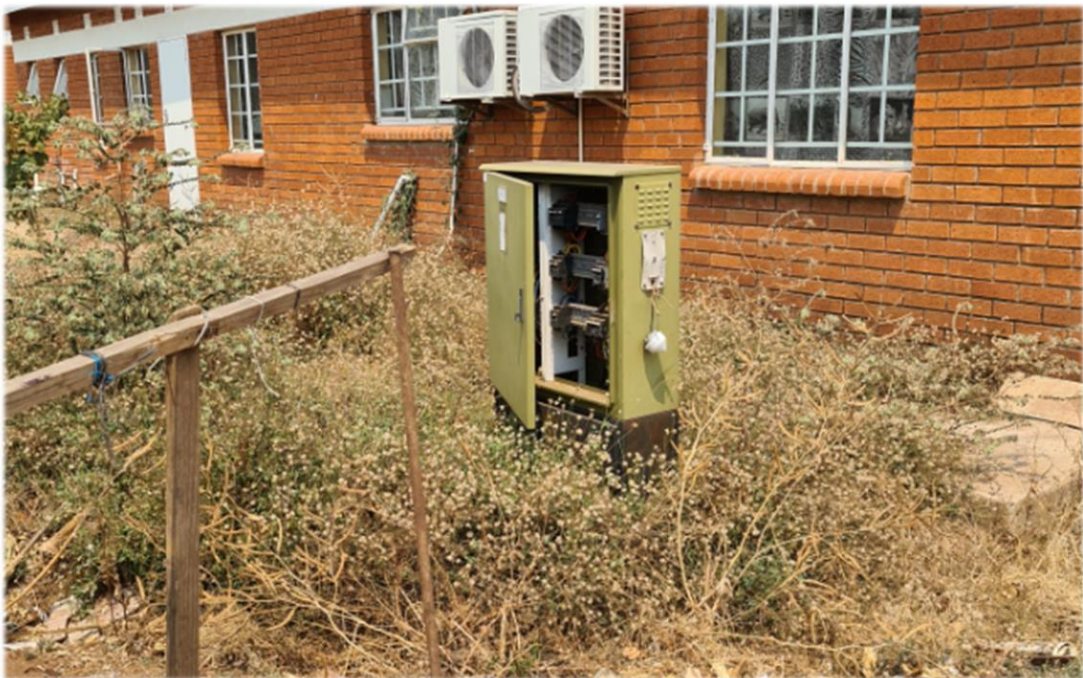
Figure 16: Vegetation Around Electrical Box
